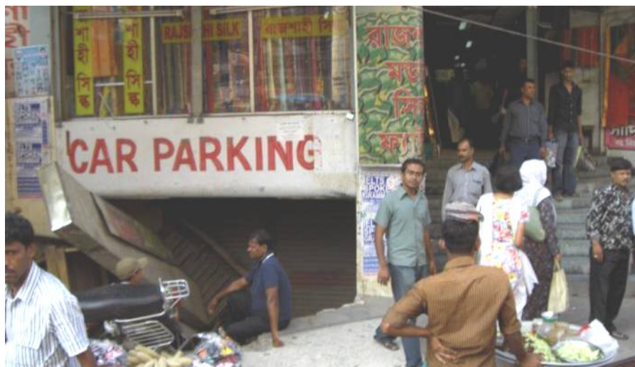
Figure 1: Basement in Dhaka presumably planned as parking space then used for shops which have now been demolished in enforcement action.
